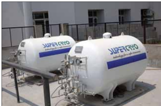
Fig. 76 2000 L capacity cryo-vessel for supply of liquid nitrogen to various repositories.
